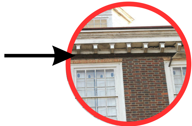
The arrow indicates the missing cornice. The shoe was discovered in this area.
