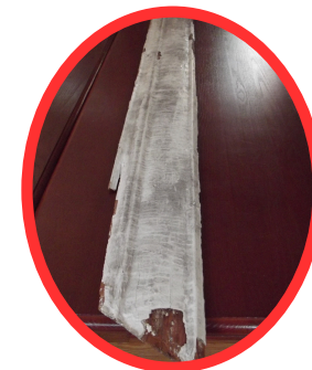
The fallen cornice is original to the house.
